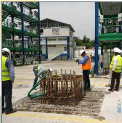
Diagnosis of cracks in a port structure in West Africa
