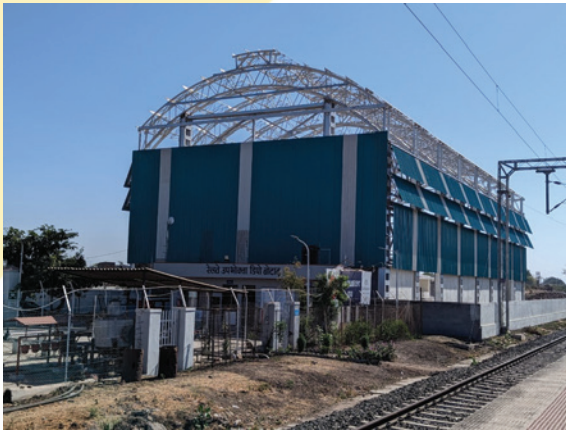
Structural Design of Inspection Shed (20m X 50m), Depot Office building and other structures.
