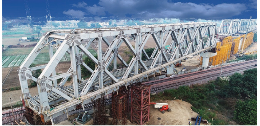
Proof checking of structural design for 142 Mtr long Railway Flyovers at ETAWAH AND BHAUPUR
